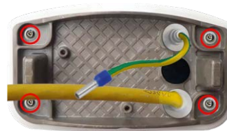
Fig. 18: Installed and ready for Connector Box LSA
